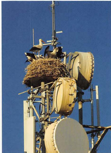
These birds in Hungary have their own ideas about the purpose of a cell phone tower.
