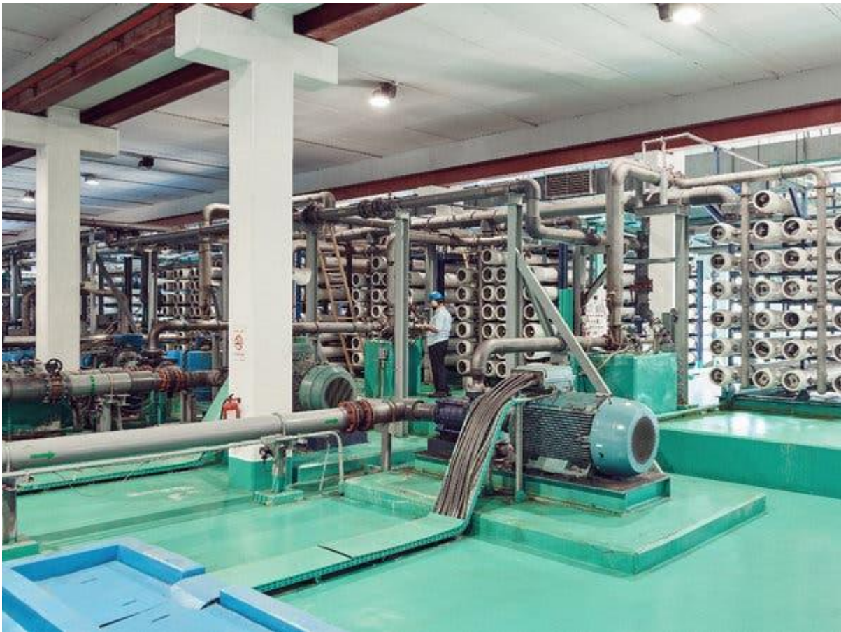
Electric water pressure pumps and reverse-osmosis membrane tubes at the Sawaco Desalination Plant in Jeddah, Saudi Arabia.
